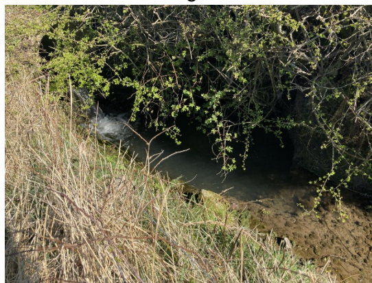
Plate 34: Unnamed Tributary of Holme Beck 9.2 (WCP_33 and WCP_34). Existing A66 culvert (A), incised channel (B and C), perched pipe culvert considered a barrier to migration for all fish species (C).
