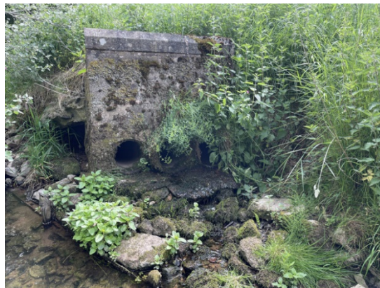
Plate 13: Unnamed Tributary of Trout Beck 4.5 (WCP_09 & WCP09). Ditch habitat, likely ephemeral (A), culvert entrance upstream of Trout Beck (B), confluence with Trout beck (C)
